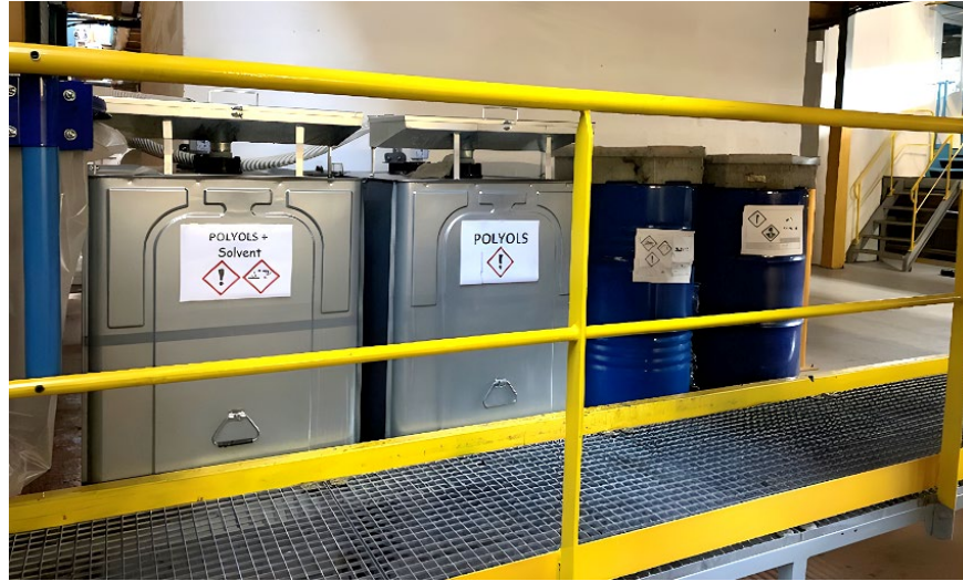
Figure 20 Dedicated waste collection infrastructure. In this facility, certain liquid waste streams are collected in fixed containers and once at a certain level will be pumped into dedicated IBCs that are moved to a dedicated waste storage location.
